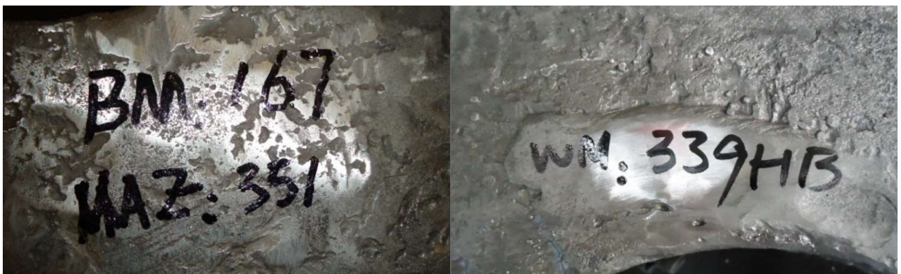
Figure 4: Defects in a casted girth gear: missed by the Contractor’s QC and spotted by the Client’s QA
